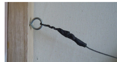
Bind dangerous exposed wire with tape
